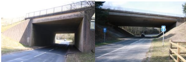
Photos 3452 and 3465 – Underpasses beneath A38 at Belvedere Cross (left) and Harcombe Cross (right)
