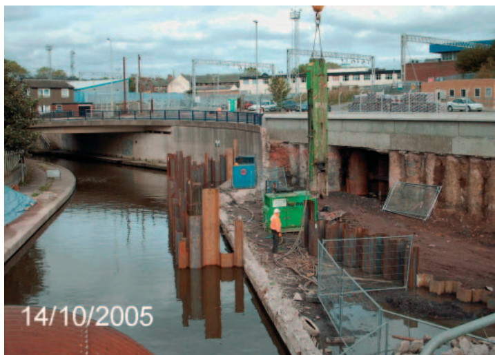
Trent and Mersey Canal - View looking north from the new Stoke Road canal bridge showing the temporary steel dam enabling work to start on the new canal basin.
