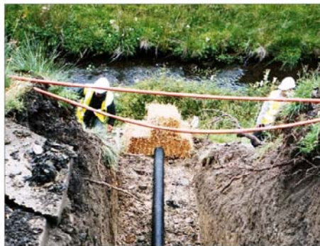
Water discharging through a straw filter to maintain water quality
