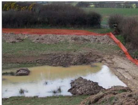
Drainage lagoon preventing polluted run-off entering a water course
