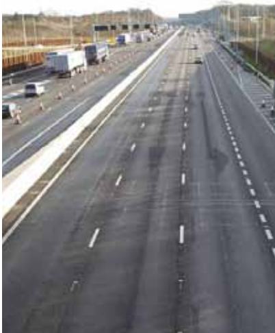
From junction 21a bridge looking towards junction 22 – the widened motorway with dedicated slip road lanes
