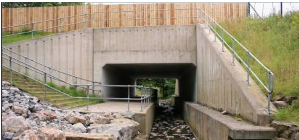
Figure G.15 - Scale Beck bridge showing footway, mammal ledge and environmental barrier
