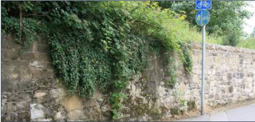
Figure G.13 - Detail of tie in between new and existing walls near the western roundabout.
