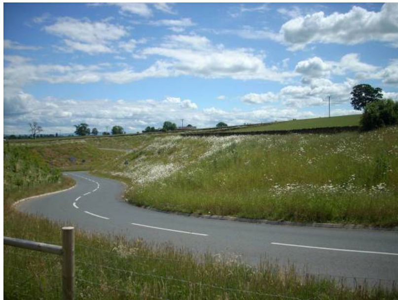
Figure C.2 – Steep slopes with extensive land drains and wildflower seeding at Cliburn Road junction
