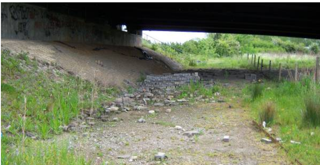
Figure B.12 Example of vandalism at north Ouse crossing
