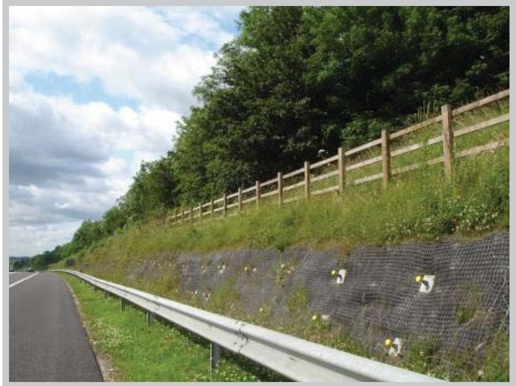
Figure I.8 - The retention of existing vegetation adjacent to the soil nailed section of ground located between Junction 31 and Vessey Close Farm
