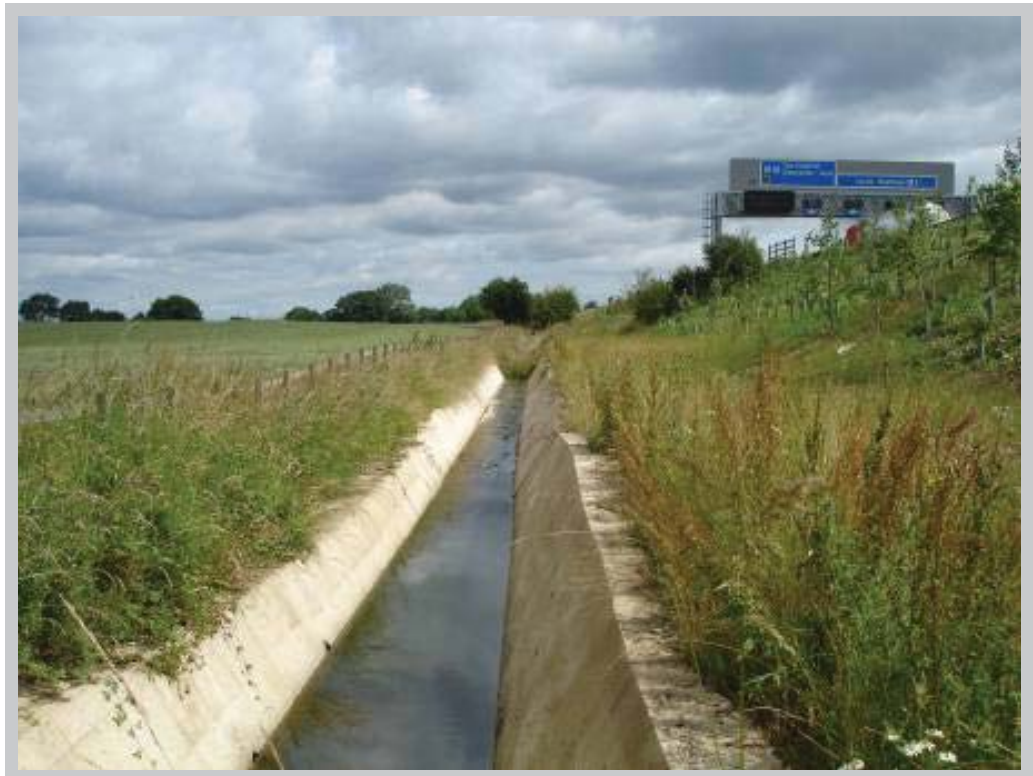
Figure I.18 - Open ditch drainage located near Ulley Beech Brook Outfall
