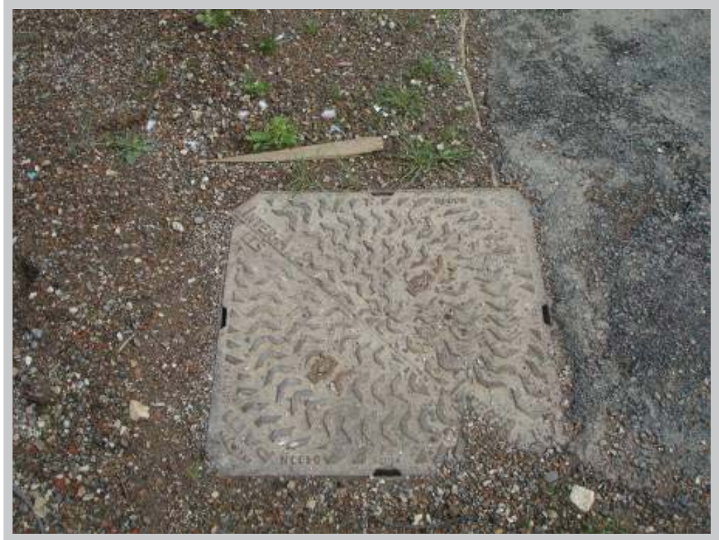
Figure I.19 - Manhole cover of Interceptor located near Ulley Beech Outfall
