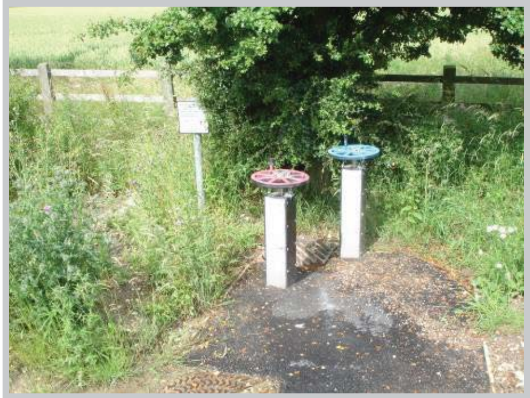
Figure I.17 - Penstock facility located at Ulley Beech Outfall
